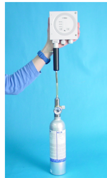
Field checking ammonia detector.
